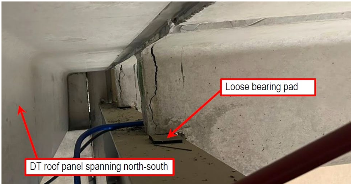
Vertical cracks at the ends of the double T roof panels. Note the roof T in the foreground has moved off of the bearing pad between it and the steel beam (Photo no. 5 from EngTech on the WM Laird Core Library, September 22, 2025).
