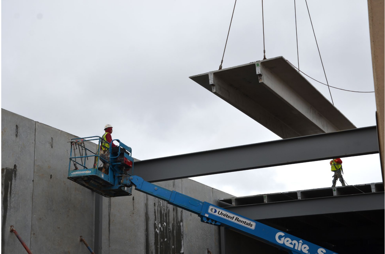
A roof panel T being lowered into place during construction of the core library expansion on March 17, 2016. The steel beams are running north-south on this part of the expansion.
