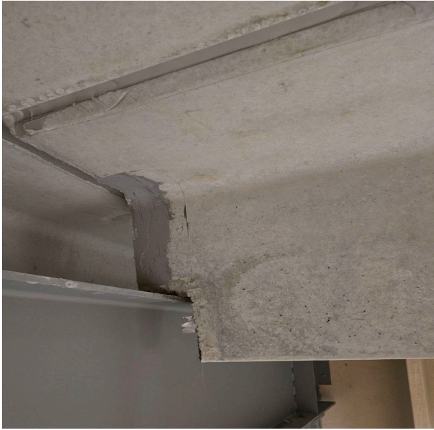
This roof panel T was welded to the steel beam and then the crack in the prefab, prestressed concrete was sealed.
