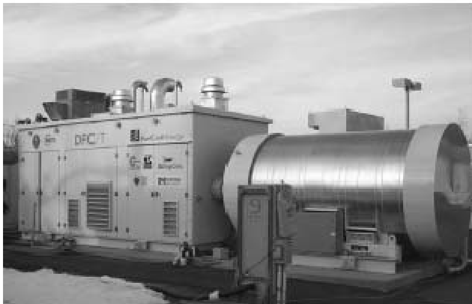
Fig. 2.4.8. The First DFC/T ® Power Plant during Factory Alpha Testing (FCE, 2009)
