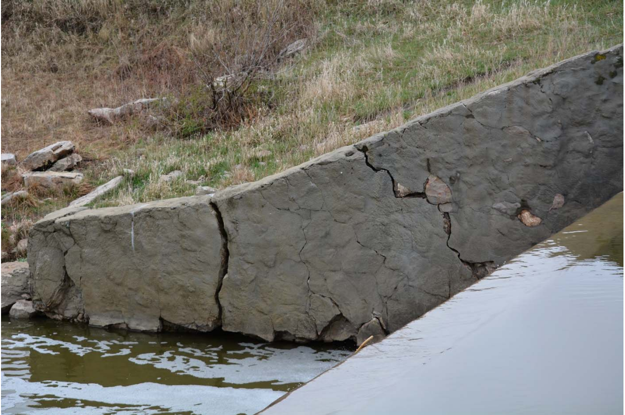
Photo 1: Karey Dam 04-26-2016 Cracking in right abutment
