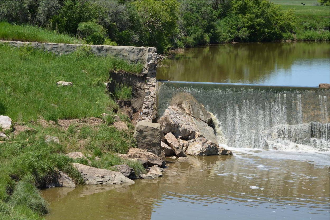
Photo 2: Karey Dam 06-08-2018 Collapsed right abutment
