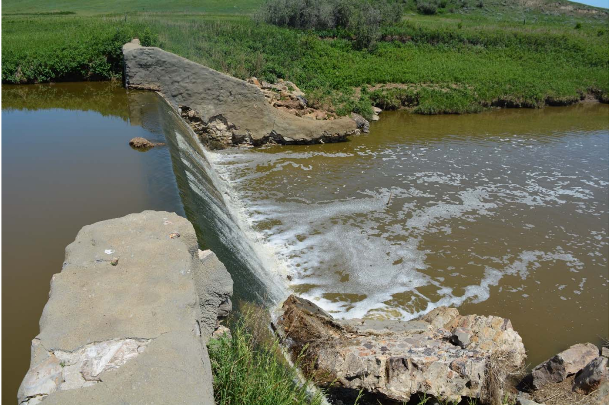
Photo 3: Karey Dam 06-08-2018 Spillway and eroded left abutment
