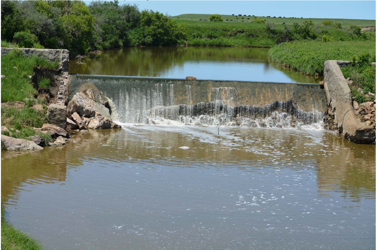
Photo 4: Karey Dam 06-08-2018 Washed out spillway and eroding / collapsed abutments
