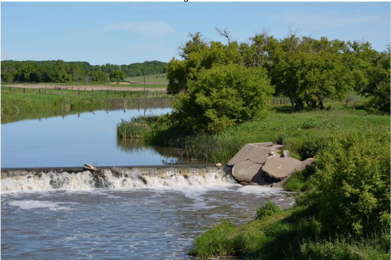
Photo 2: Bouret Dam 06-07-2016 Eroded left abutment and washed out spillway
