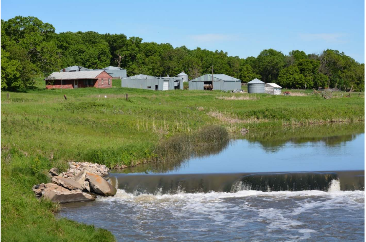
Photo 1: Bouret Dam 06-07-2016 Washed out right abutment and loose boulders
