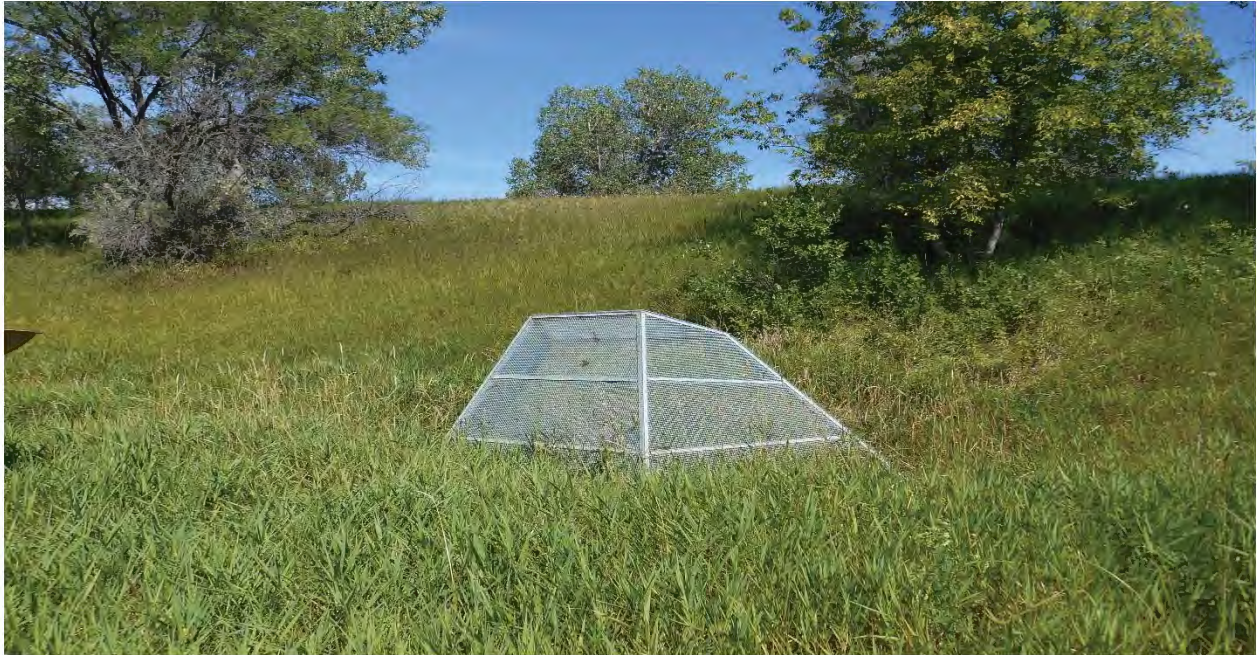
Debris Screen For Existing 24-Inch CMP at 4-H Camp
