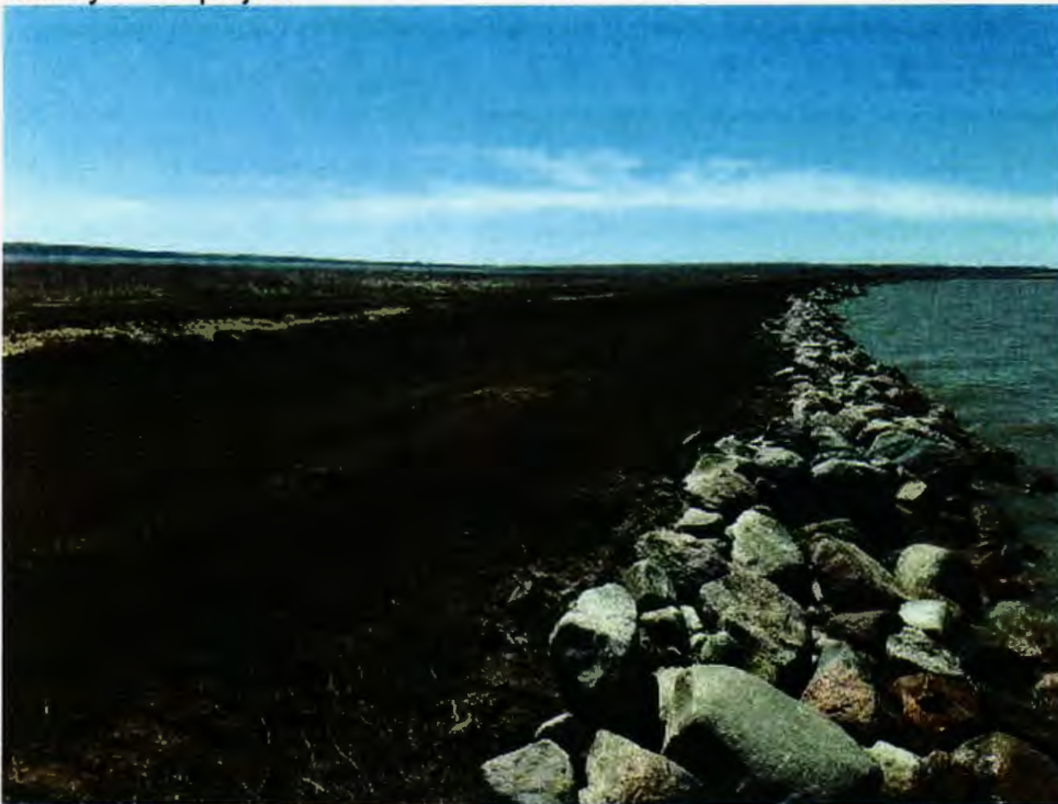
Nearing completion of the 5,000 feet of raising the embankment, filling breaches, and armoring the face of the lake to eliminate erosion and protect the restored 444 acre Unit II marsh behind it.
