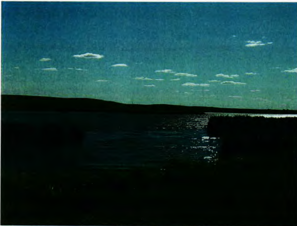
Alkali Creek wetland impoundment after pipe installation and rip-rap armoring of eroded embankment.
