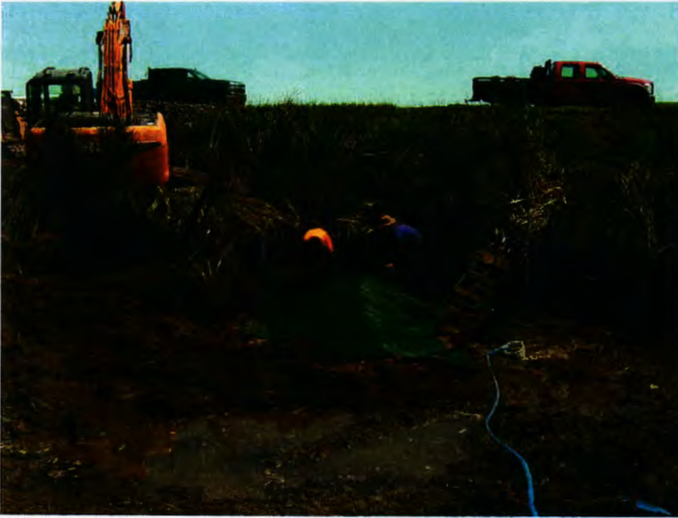
A new perforated pipe being installed at the 58-acre Alkali Creek Wetland Impoundment project so that sediment does plug the water control structure.
