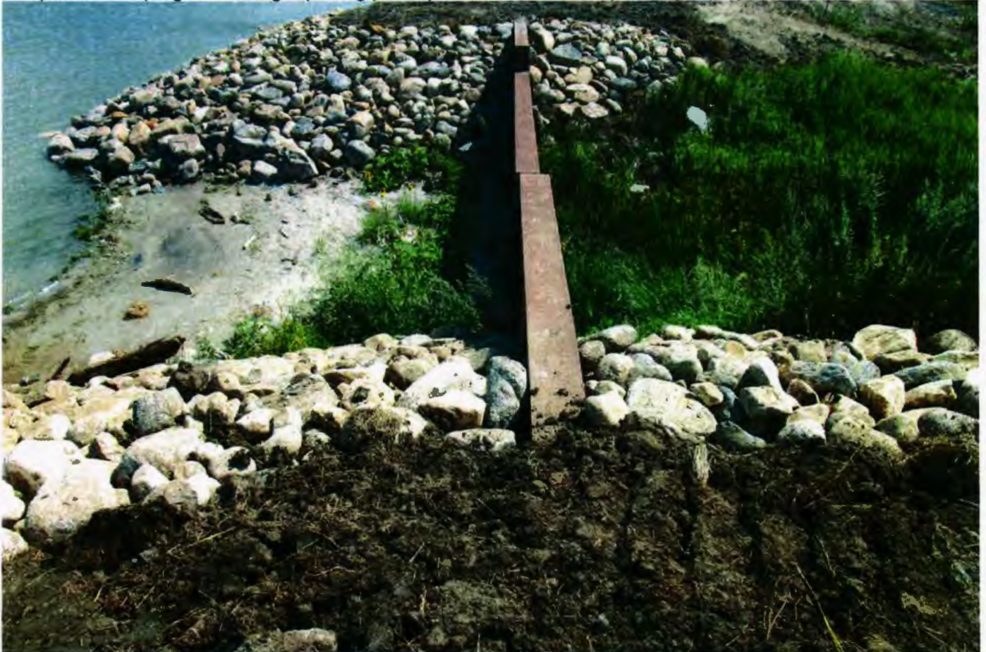
The completed G-19 project with newly armored embankment and water control structure that restored 10 acres of emergent wetlands previously drained by bank erosion.
