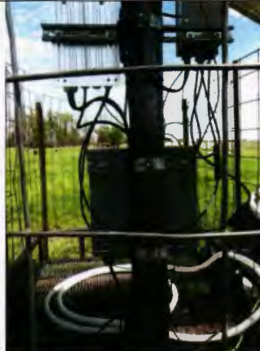
The solar trailer with protective paneling around it
