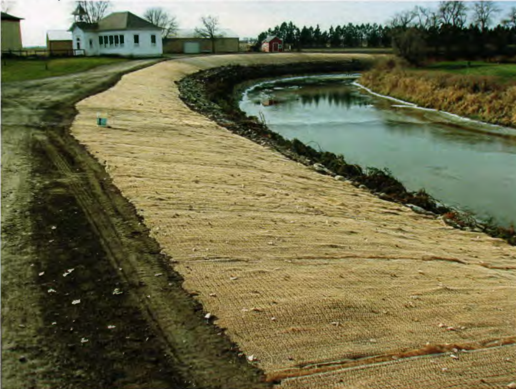
Revegetation of the disturbed slope and erosion fabric installation The completed Crib Wall can also be seen here
