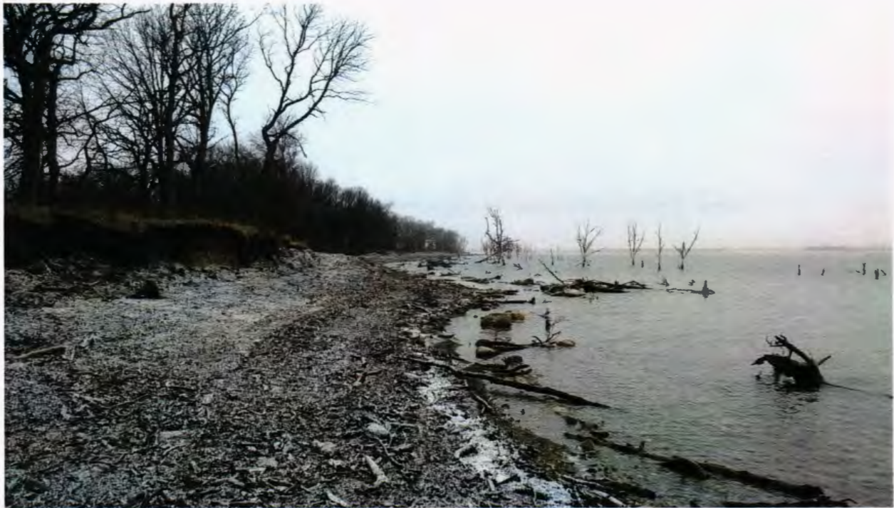
Washout shoreline before restoration
