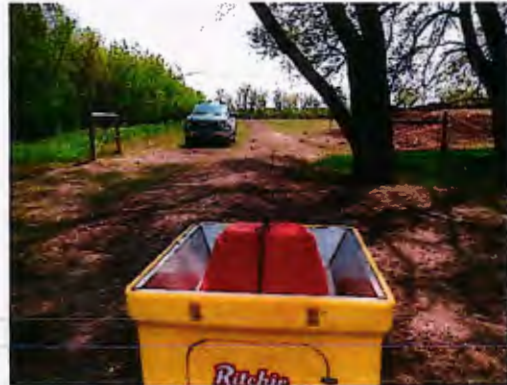
600 foot pipeline with watering tank to facilitate cattle rotation.
