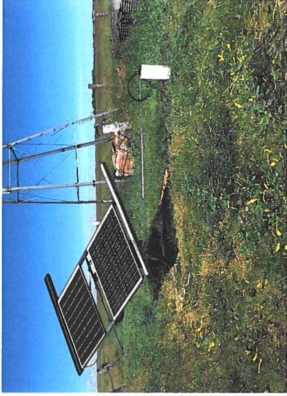
Solar Pump for Well
