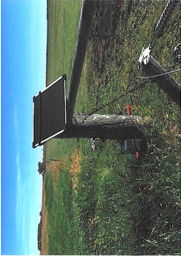
Electric Fence Solar Generator
