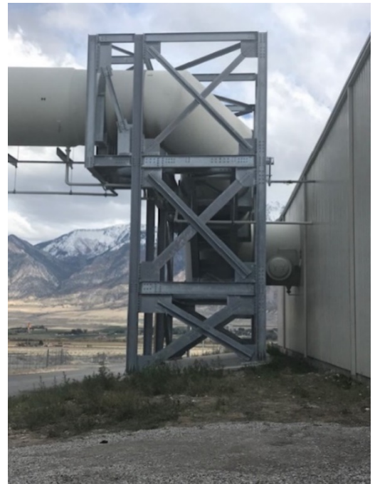
Connection piping into Utah greenhouse
