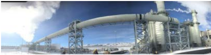
Connection piping between Utah greenhouse and power plant
